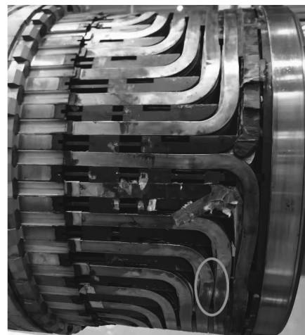
图7 转子绕组端部存在顶匝变形现象 Fig.7 Top turn deformation phenomenon at the end of the rotor winding
